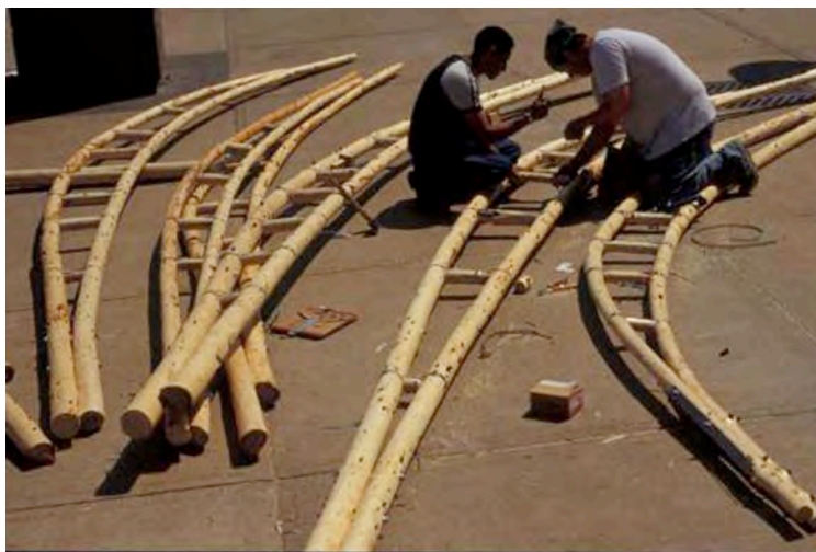
Figure 5: Murdena Marshall Meeting Hall, Cape Breton, Nova Scotia, assembly of small dimension lumber thinnings into structural members (photo: Richard Kroeker).
